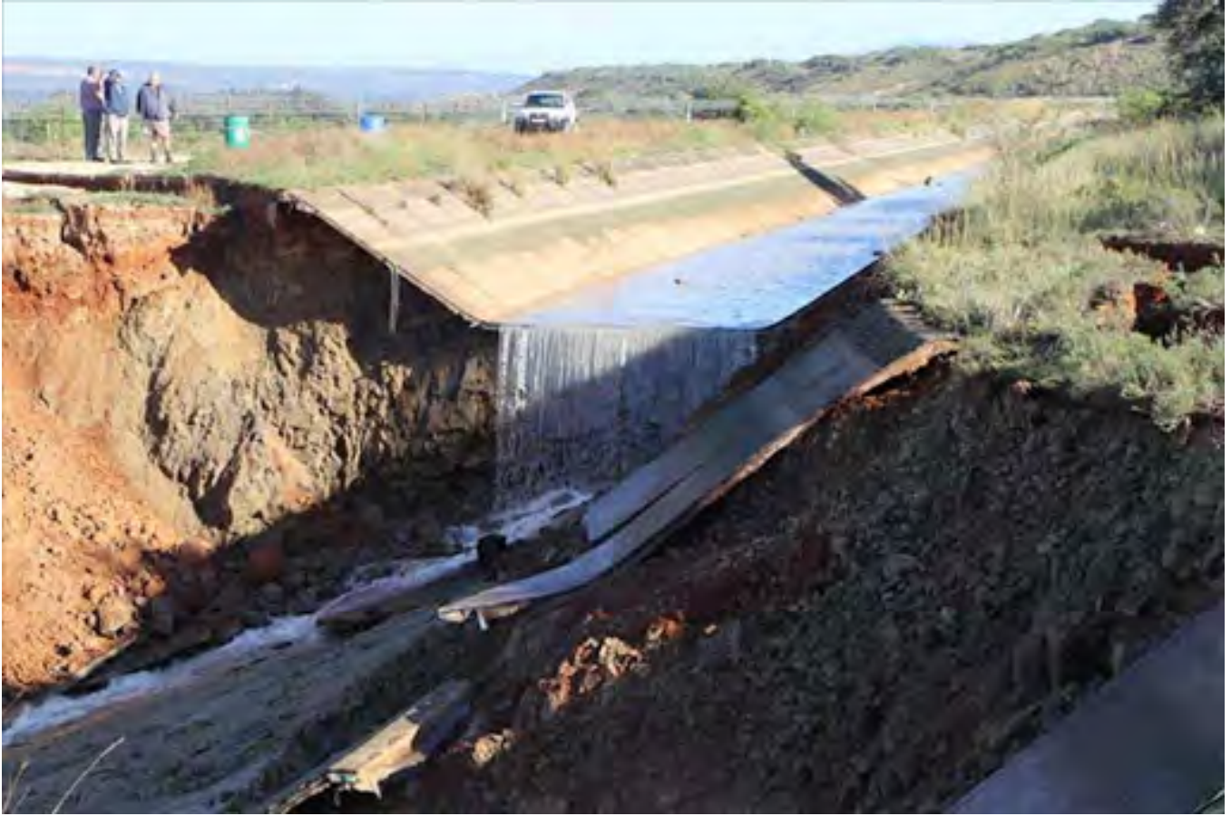
Figure 4-8. Damage to the Kirkwood Canal supplying water to the Algoa Water Supply System in 2017, Picture: Riaan Marais 28
