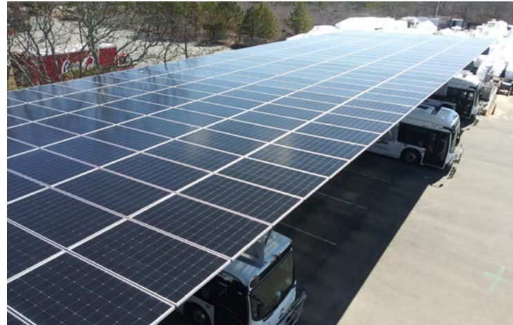
4: The 700kW DC solar PV array at the bus depot provides clean, renewable and cheap energy 5: VTA's microgrid pairs battery storage with its solar energy system
