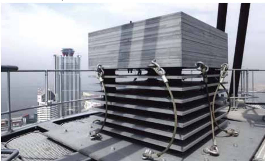
56. Tuned mass dampers.
