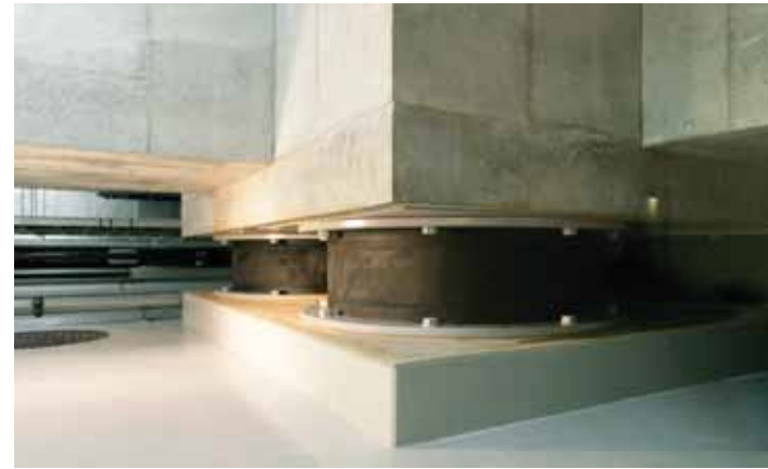
63. Close-up of rubber bearings.
