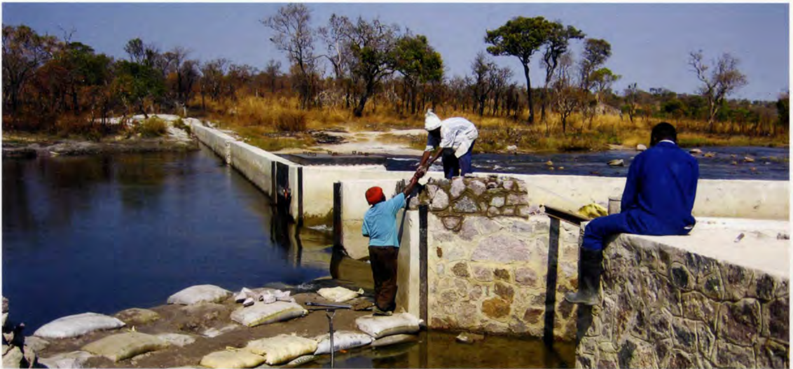
5. The weir under construction, showing the automatic sluice gate in the centre, and fitting gate channels to the entrance to the canal in the foreground.
