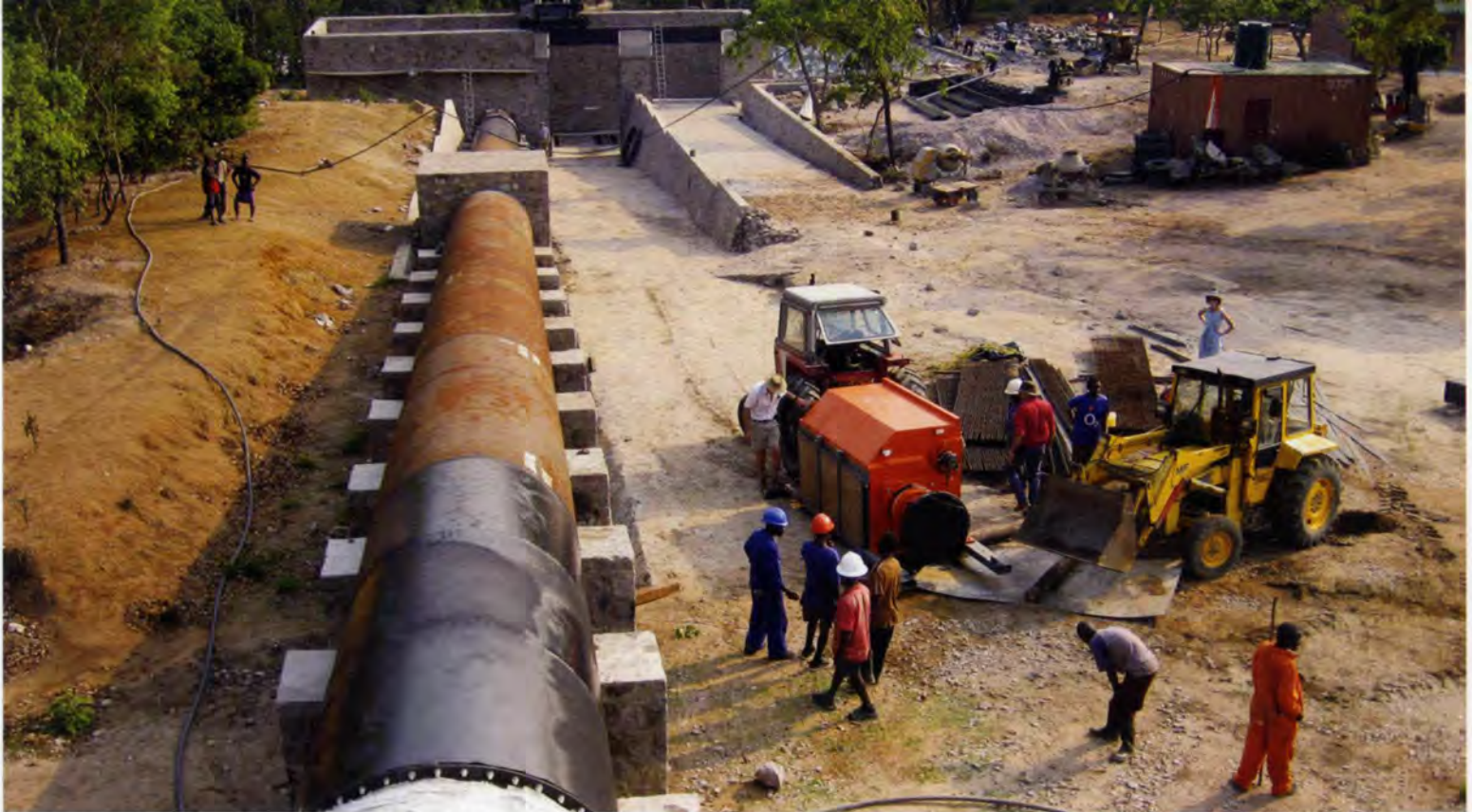
1. Not everything can be done by manpower - dragging the 700kW turbine for installation in the powerhouse.
