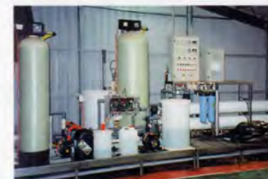
5. Reverse osmosis equipment.
