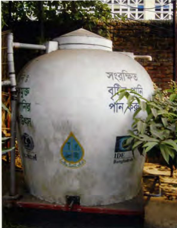
2. Rainwater harvesting system.
