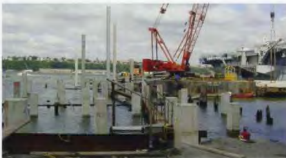
12. New hybrid precast prestressed piling for Pier 84, Segment 6, threaded amongst the remains of the old timber piles.
