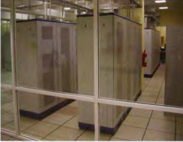
9. The main server room.
