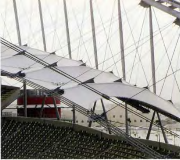
12. Main roof catenary and ridge clamps.
