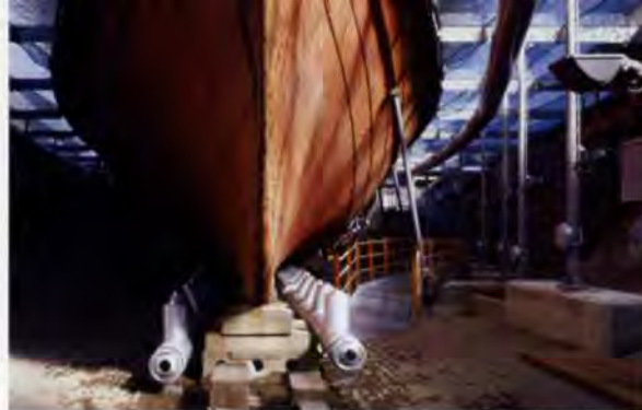
3. Low level dehumidified air supply and high level extract ductwork at the bow.
