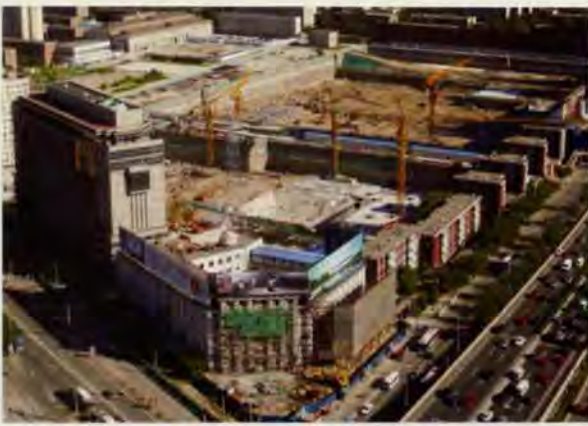
9. Site progress, August 2005: TVCC is in the foreground, with piling completed and excavation to the base of the rafts. Piling is complete at CCTV (behind) with excavation under way to the base of the rafts (up to 30m below ground level).
