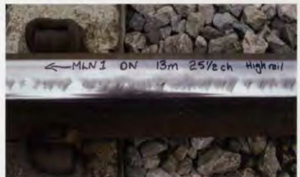
4. Head checking on a 1300m curve.
