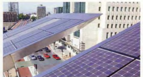
6. PV cells on upper surface of cantilevers.
