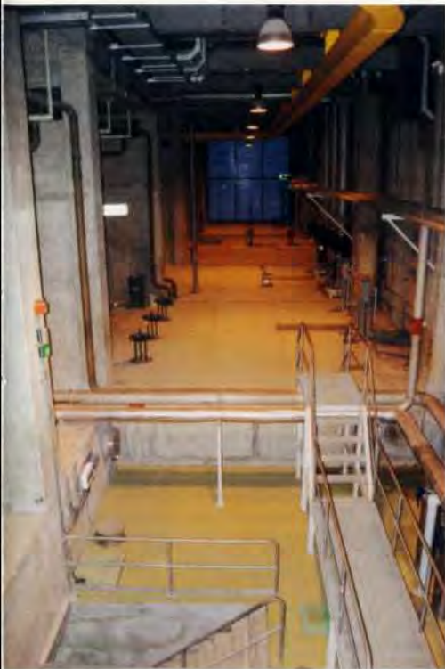
19. Central gallery of treatment plant.
