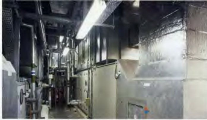
13. Air handling plant at level 1.
