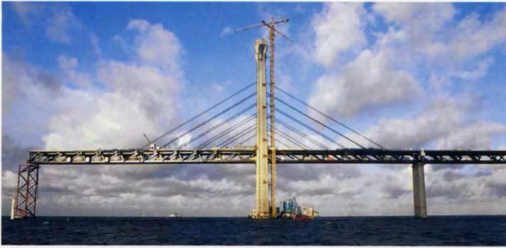
20. The main span was erected in four sections supported by temporary towers.
