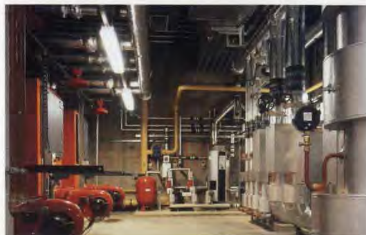
15. Central boiler room.
