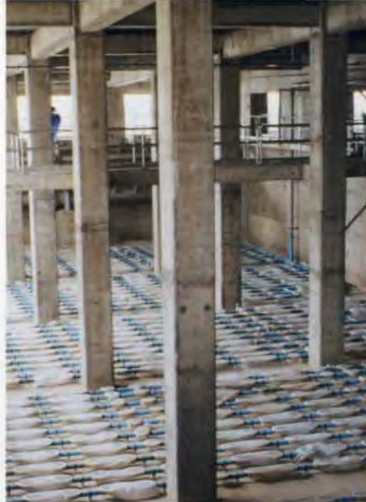
13. Treatment basin, showing bubble aerators.
