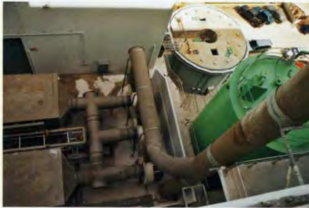
15. Chemical scrubber for odour control.
