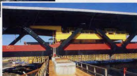
10 below: The lower deck in the approach girders was completed in the Malmö yard.
