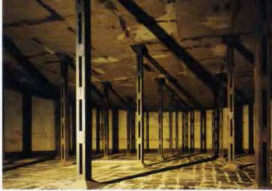
19. One of three similar chambers which contained oil tanks for the power station. These may form a future phase of Tate Modern.
