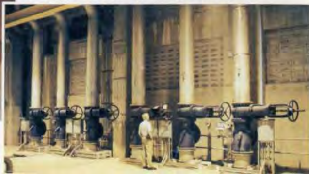
11 below: Delivery pipes from CASS™ pump station in central gallery.
