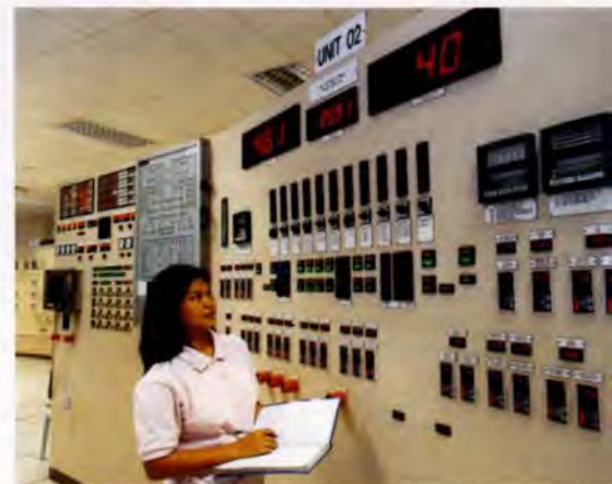
12. Central control room.
