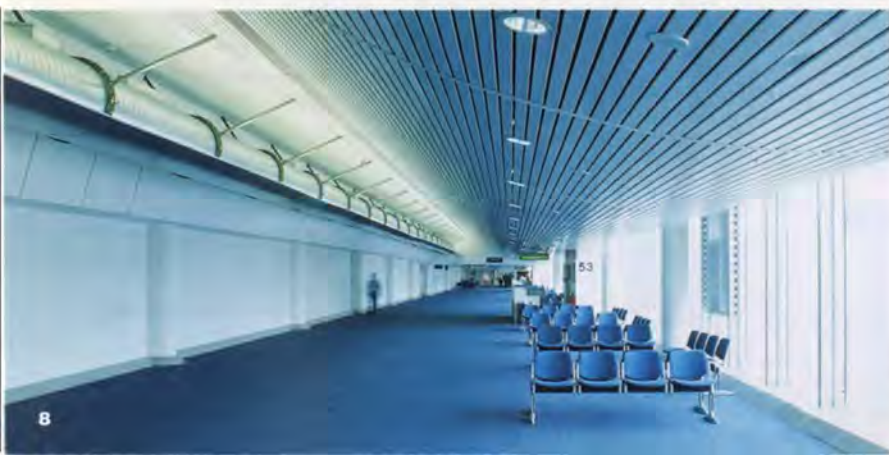
14. Co-ordinated mechanical and electrical services in international departure pier, T3.
