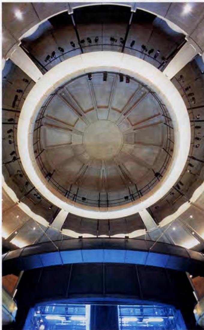
7. Auditorium roof showing use of structural ribs for sound diffusion and 'jelly-mould' sound diffusing form of vertical precast sections.
