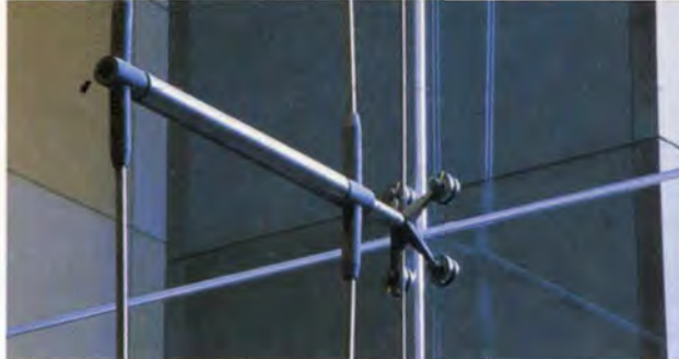
12. Screen truss strut and connection detail, showing 19mm truss rods and 9.5mm glazing rod.
