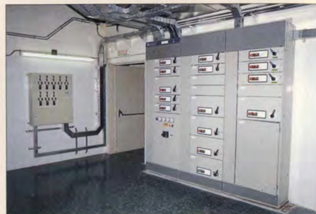
B. Chiller (motor) control centre.
