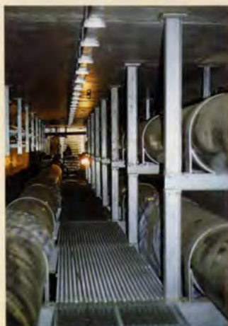
B. Condenser cooling pipework in box culvert leading to seawater pumphouse.
