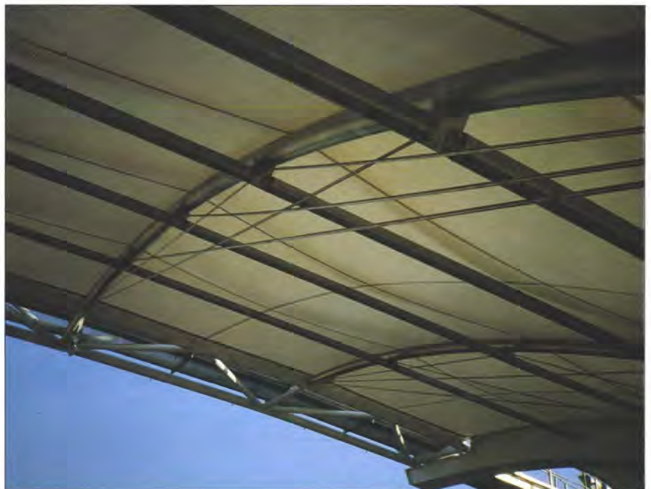
6. Under the canopy roof, showing stainless steel tubular arch-beam with stabilizing chord-ties
