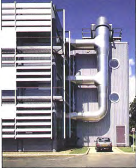
7. End view showing pods, ducts, etc.
