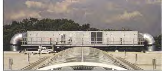
12. View across the roof of one air-handling unit, supported on a gantry above the roof surface.
