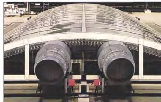
14. Close-up of two smoke extract fans on the roof.
