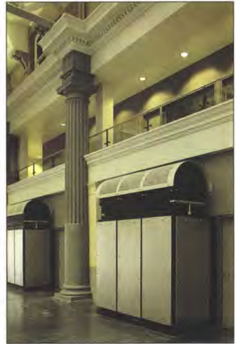
15. Free-standing AHU on ground floor
