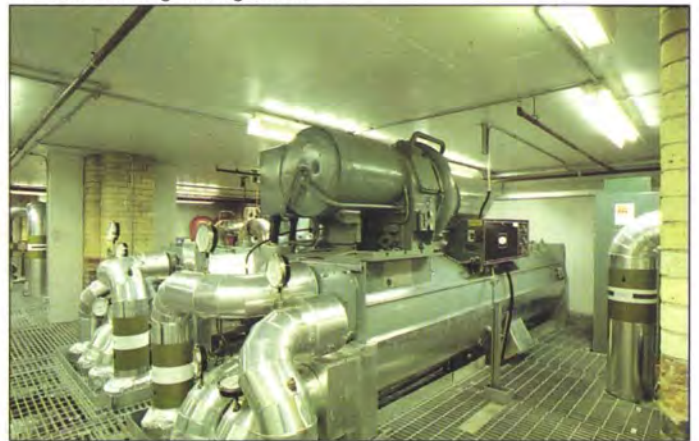
21. Chiller plantroom north-east corner
