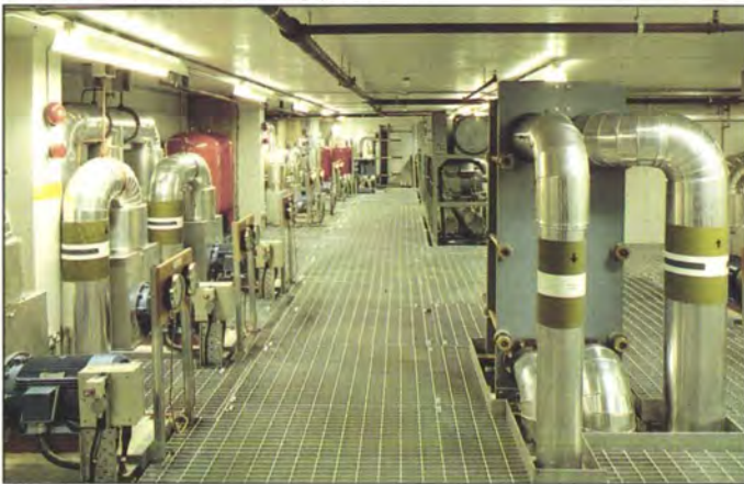
20. Chiller plantroom facing east
