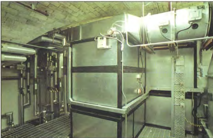
18. One of the 15 air-handling plantrooms
