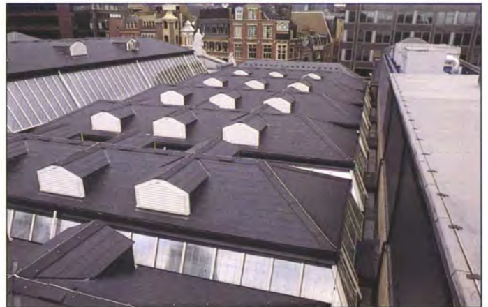
19. Roof showing cooling towers
