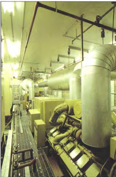
16. Diesel generator room
