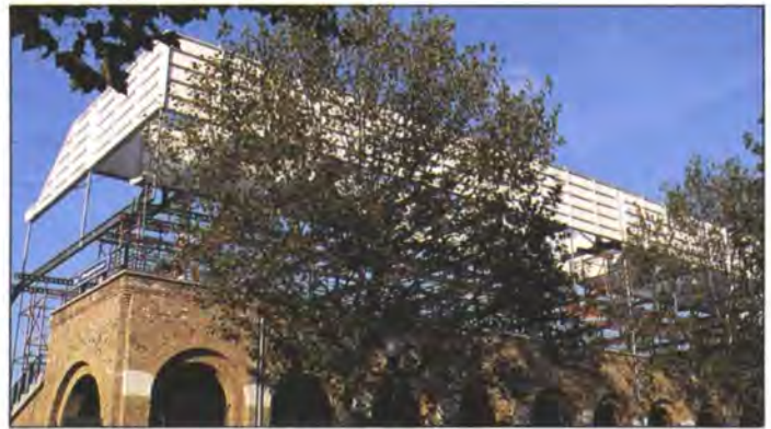
3. The beam system during construction showing the new brick arches (Photo: Harry Sowden)
