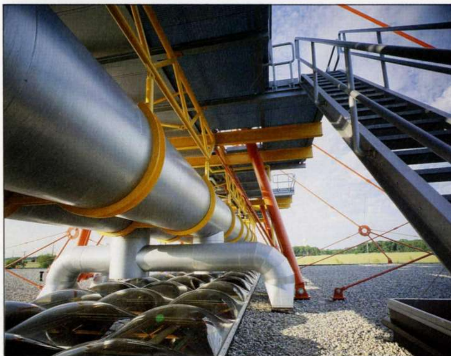
19. Primary ducts above spine skylight with connections to lateral feeders in research enclosures (Photo: Otto Baitz)
