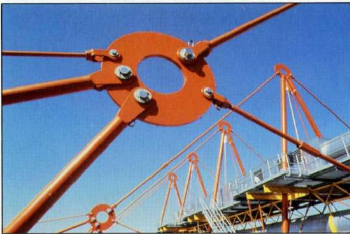
20. Annular node plate of suspension system, looped tapes for continuity of lightning protection can just be seen (Photo: Barry Dunnage)
