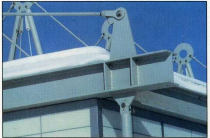
21. External view of corner during construction, again showing looped tapes for continuity of lightning protection (Photo: Ram Ahronov)
