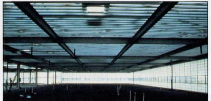
14. Left: Interior view of Kalwall cladding during construction 15. Above: General interior view of research enclosure, prior to casting ground slab or installation of services, showing column-free interior and transluence of Kalwall cladding. (Photos: Ram Ahronov)
