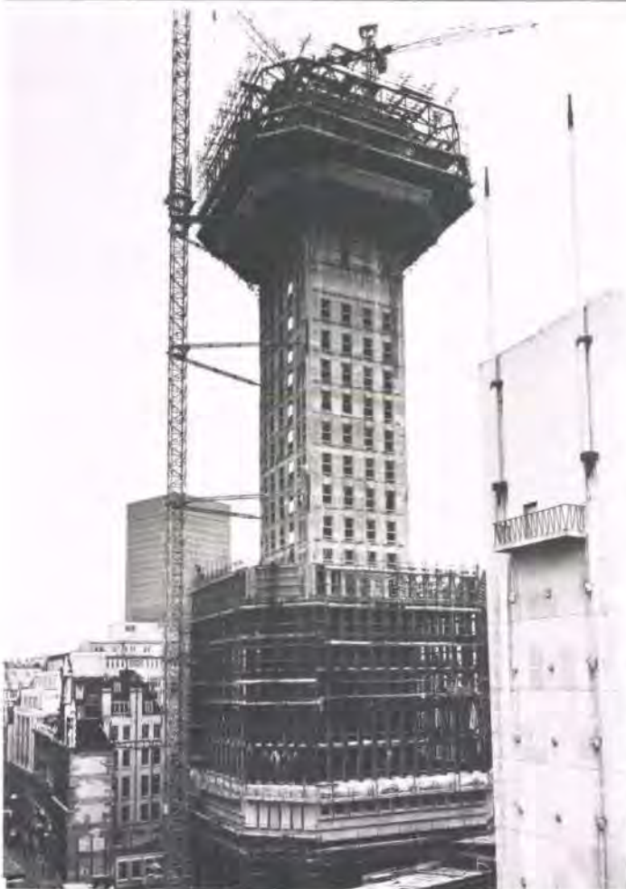
The slipformed core of Barclays Bank Chief Foreign Branch, London EC3 (1969-72) Architect: City of London Real Property Co. Ltd. (Photo: W.H.R. Goodman)
