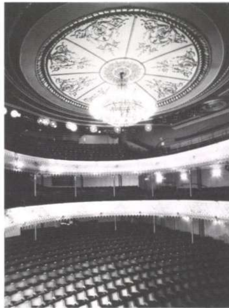
Fig. 13 Auditorium and galleries. Supply air diffusers encircling ceiling rose
