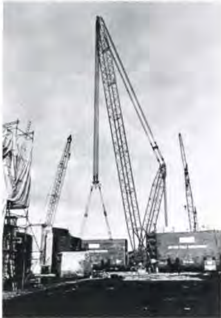
Fig. 4 Pontoon section being lifted into position during assembly at Hutton TLP lower hull at Nigg
