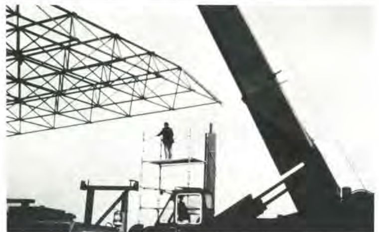
Fig. 5 Bailey's Irish Cream factory: lifting the space frames. Architects: Scott Tallon Walker
