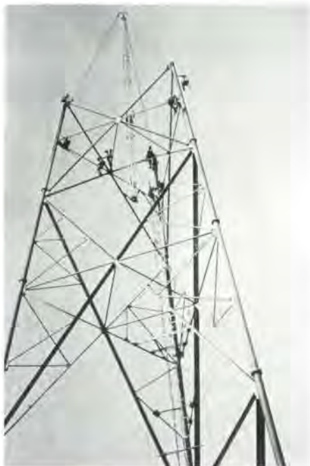
Fig. 3 Microwave tower under construction in Nigeria, designed by Ove Arup & Partners (Photo: Mike Shears)
