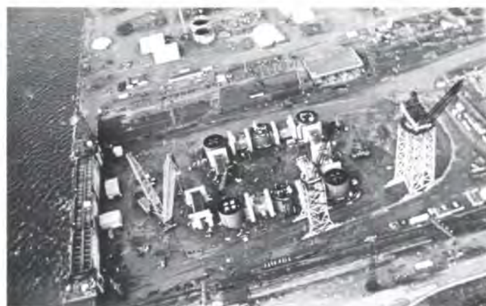
Fig. 3 Hutton TLP tower hull under construction in the dry dock at Nigg. Pontoon is about to be lifted in.
