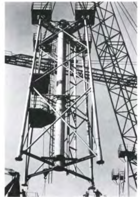
Fig. 5 Brent C flare tower: erection of tower sections (Photo: courtesy of Sea and Land Pipelines)
