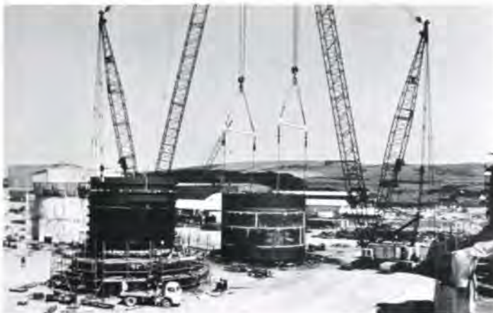
Fig. 5 Hutton TLP column under assembly at Nigg. Outer shell about to be lifted over inner shell to form splash zone double skin 'damage control' section
