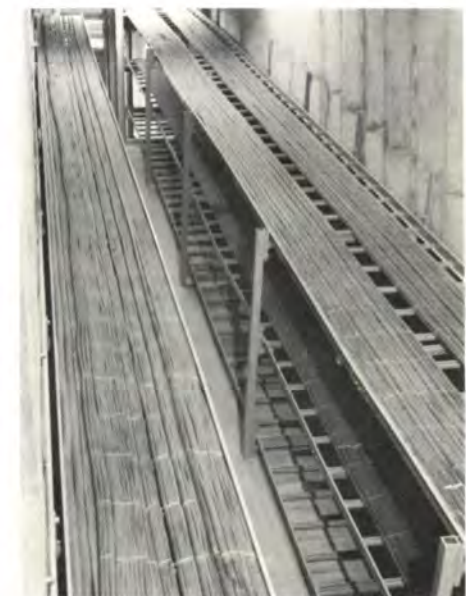
Fig. 30 Cable access to sub-basement (below MCCs)
