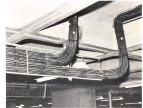
Fig. 29 Typical cable racking, below main floor coffered slab
