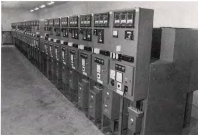
Fig. 40 31 panel 11kV main switchboard
