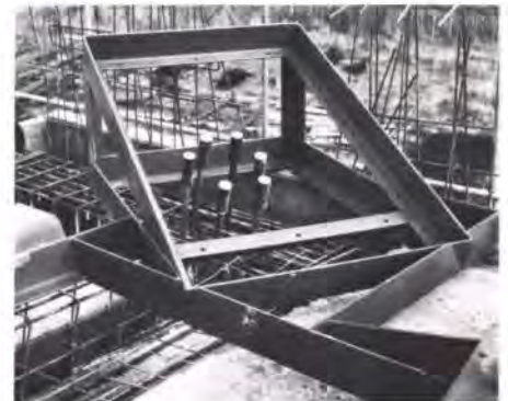
Fig. 15b Corner of template showing backtie connection detail (Photo: copyright Greater London Council)
