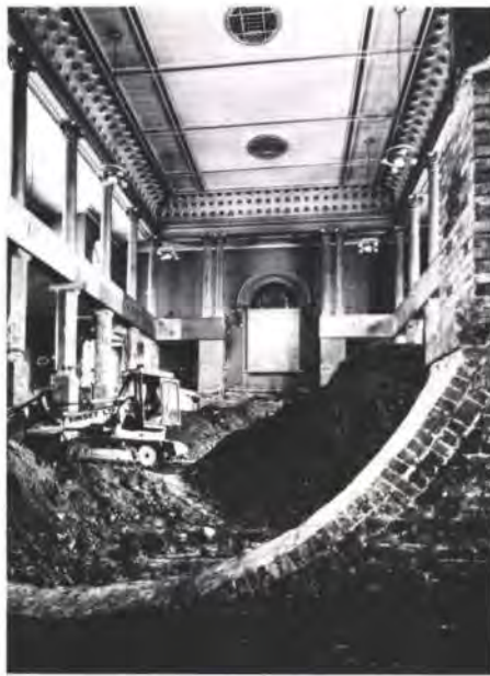
Fig. 1 Excavation in progress seen through wide inverted arch at west end (Photo: Thomas-Photos)
