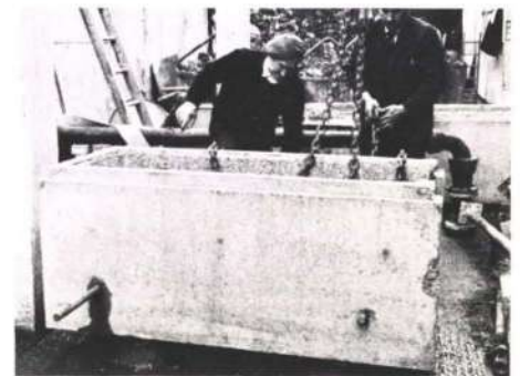
Fig. 5 Precast column foundations being jacked down on top of bearings. (Photo: Mark Gerson)
