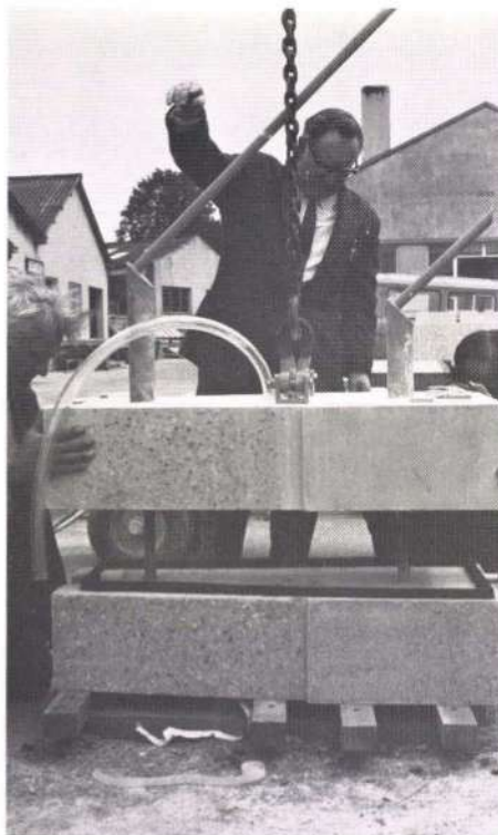
Fig. 6 Full scale 'mock up' of typical joint between precast columns (Photo: Ove Arup & Partners)
