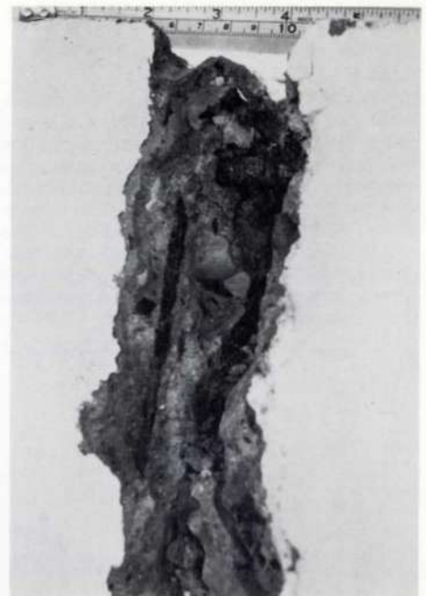
Fig. 2 Close up of top of crack in roof beam
