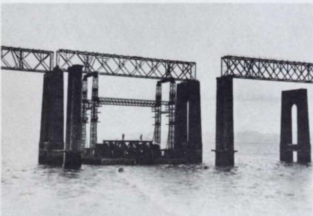
Fig. 4 above Lifting the remaining girders off the old brick piers for re-use in the new bridge. The new double-leg piers contrast with the narrow height of the old single-line bridge.
