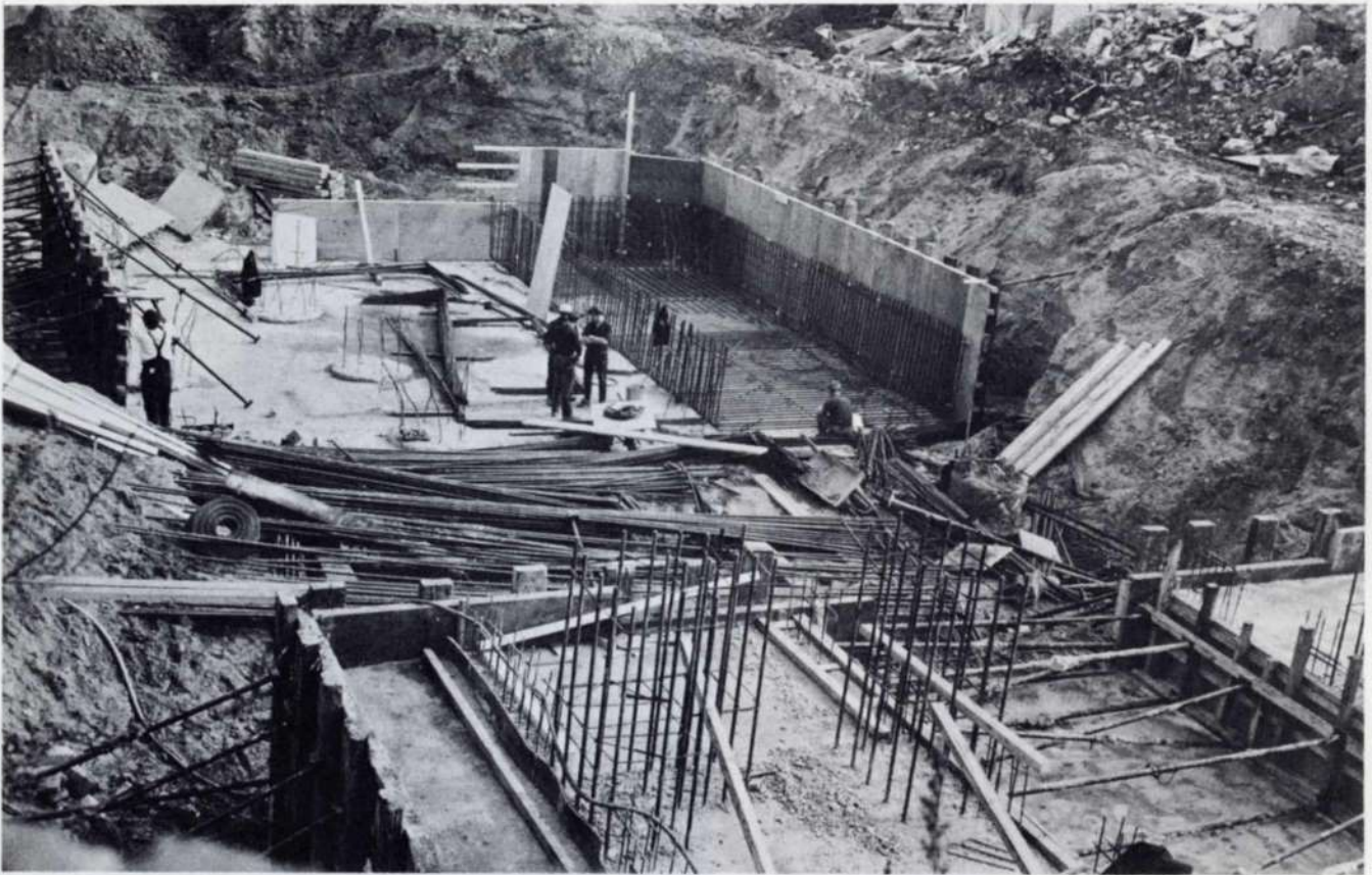
Fig. 3 300 cubic yard pour in course of preparation. In the foreground a completed 300 cubic yard pour.
