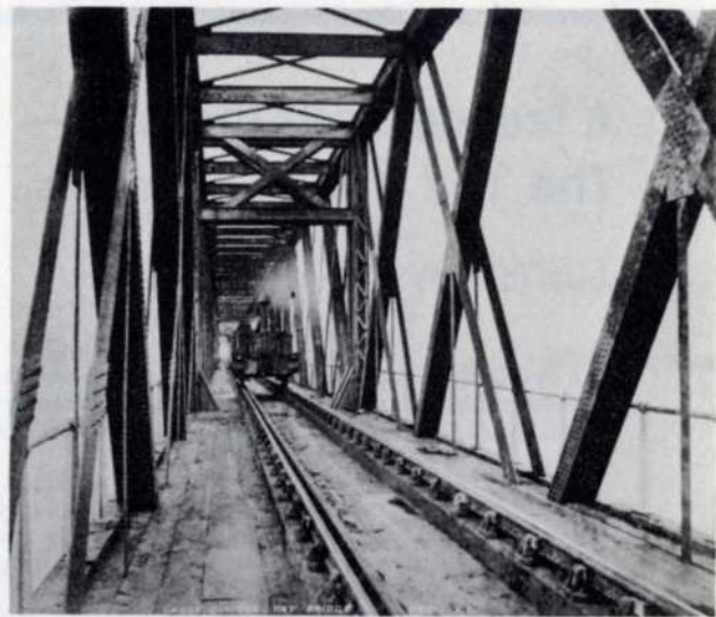
Fig. 1 Engine inside the navigation spans of the old Tay Bridge. Tie members are unbraced flats with unusual rivet pattern of horizontal rows.
