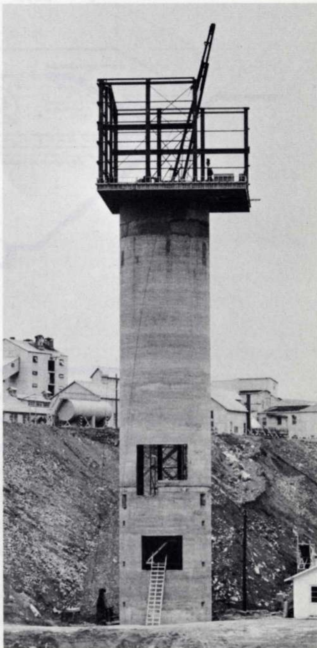
Fig. 1 View of tower during construction of penthouse before backfilling to underside of upper opening. (Photo: Leigh W. Bladon)
