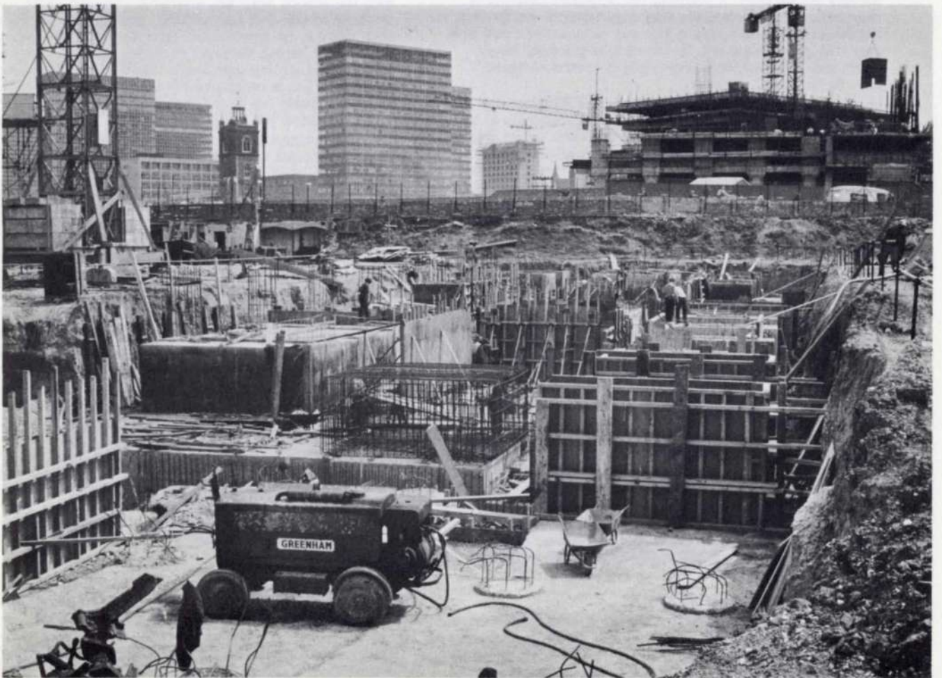
Fig. 2 below General view of Block 14, Barbican Redevelopment, showing pile caps in various stages of construction.
